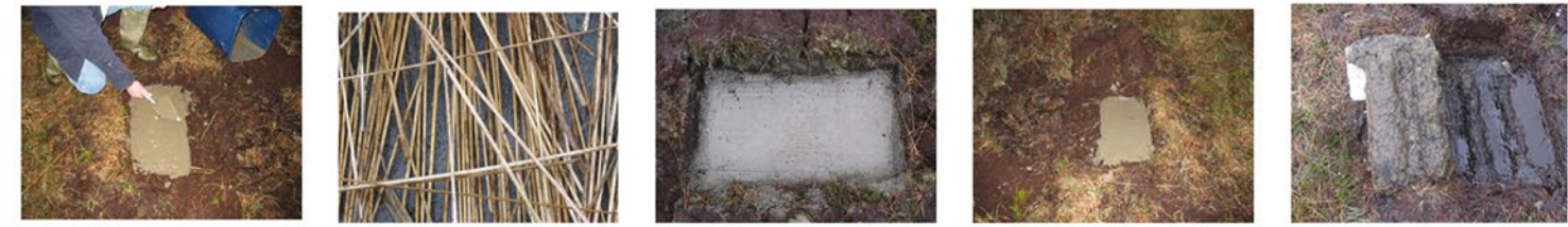
THE CONCRETE TOOK 3-4 DAYS TO SET PROPERLY, WITH THE BOTTOM OF THE SLAB DRYING QUICKER THAN THE TOP.
