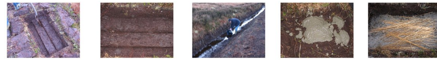
THE DIMENSION OF THE THE SLAB POURED WAS . 500X400X 250MM THE MIX CONTAINED SAND, FINE AGGREGATE, CEMENT AND BOG WATER. I USED VARIOUS MIXES BUT A DRY MIX SEEMED TO SURE THE CONCRETION IS BETTER.
